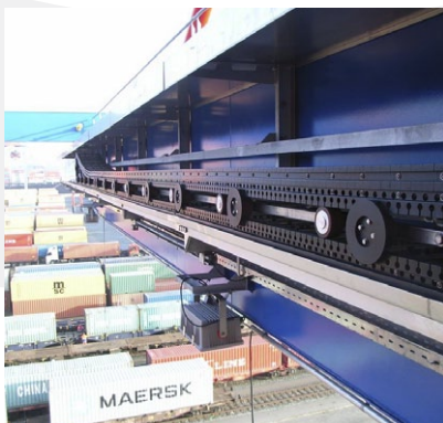
Energy guiding chain solution for trolley – Railway terminal, Weil am Rhein, Germany
