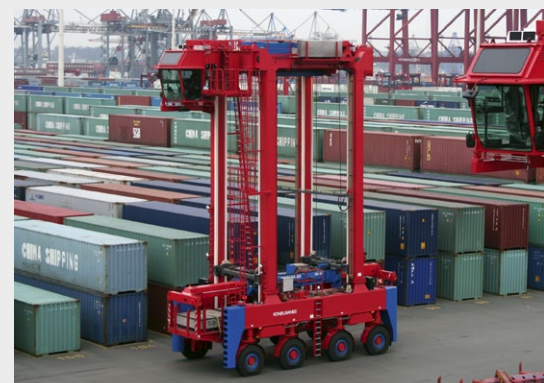
Cable chain system on a straddle carrier – Hamburg, Germany
