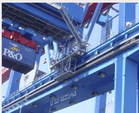
Cable chain system on a trolley – Hamburg, Germany
